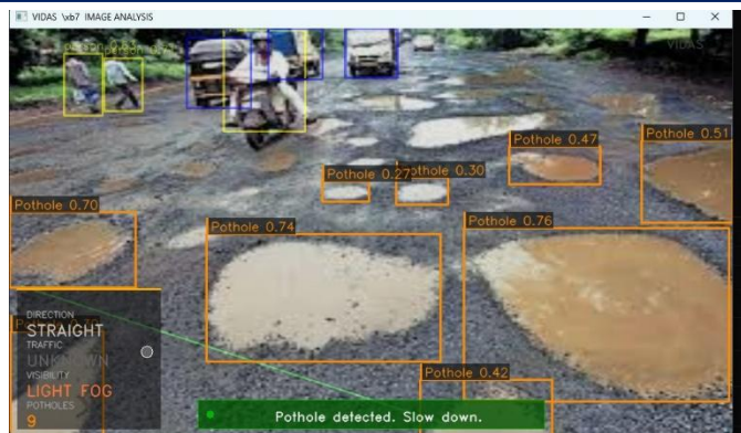
Fig. 6: Pothole detection using a custom-trained YOLOv8 model.
